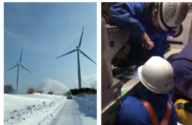
Testing on real wind turbines was conducted in the Central Hokkaido area, with the team entering the turbines and ascending 70 to 80 meters to install the testing units
