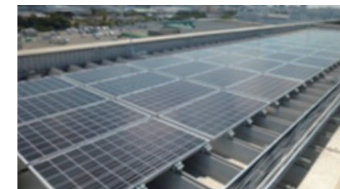
Solar panels installed at the Kobe Plant
