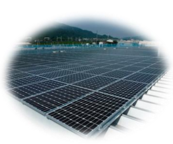
2012 Tarui Plant 400kw
