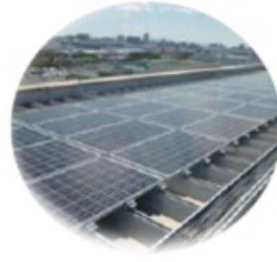
2016 Kobe Plant 500kw
