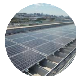
Solar panels at Kobe plant
