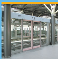
Platform screen doors
