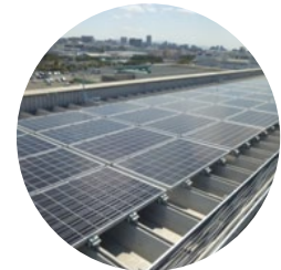
Solar panels at Kobe plant
