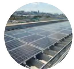
Solar panels at Kobe plant
