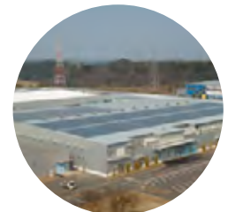
Solar panels at Tsu plant
